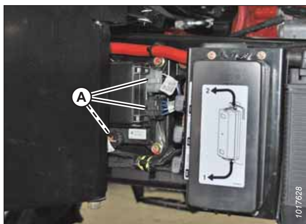
Figure 1.25: Chassis Relay Module
