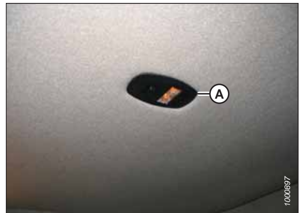
Figure 6.177: Ambient Light Fixture
