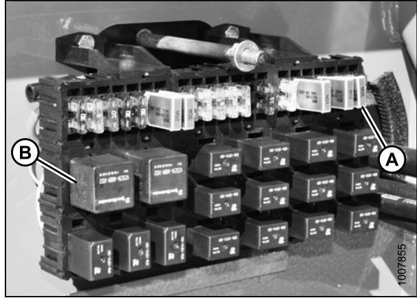
Figure 5.168: Breakers and Relays
