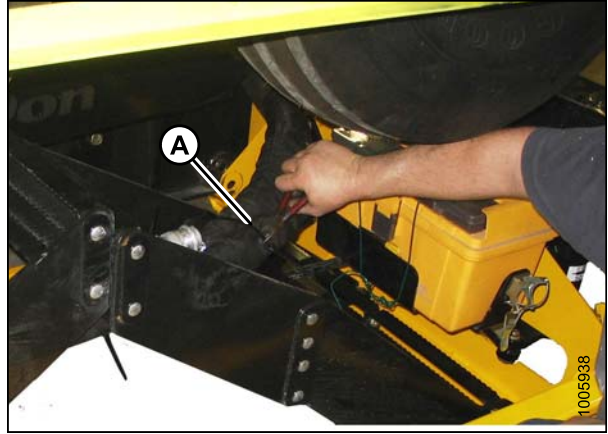
Figure 2.12: Hose Bundles on Frame
