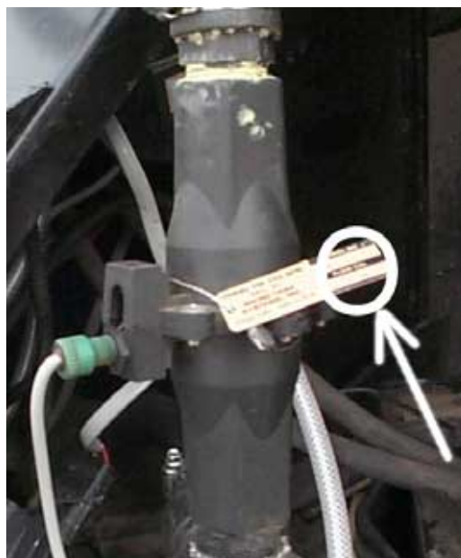
Calibration tag attached to the Flow Meter.
