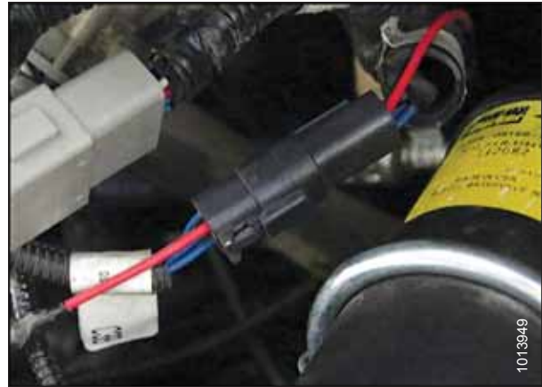
Figure 3.28: Harness Connected to C3B
